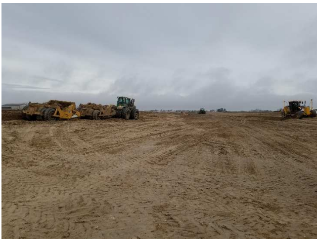
Cutting P-152 fill material from borrow area on South side of the runway.
