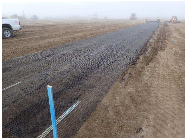
Placing geo-grid material on surface of P-152 in soft spots along runway alignment.
